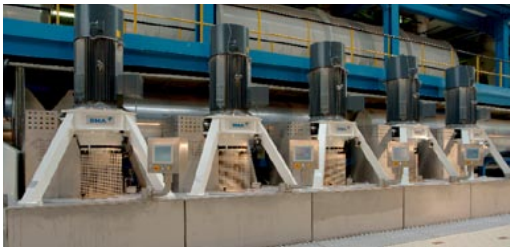
Centrifugal station with B1750s
