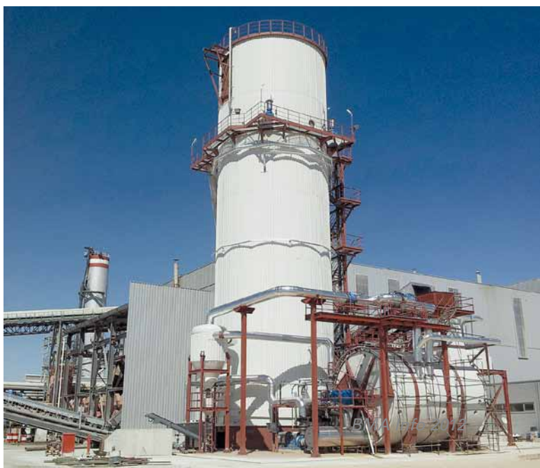
Extraction plant at the Kesinkili  sugar factory
