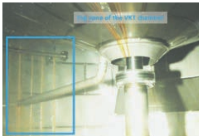
Fig. 5: Ring pipe with feed solution for wall cleaning
